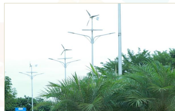
Solar and wind powered LED street lights
