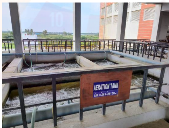
Sewage Treatment Facility (STP) at VIT Chennai
