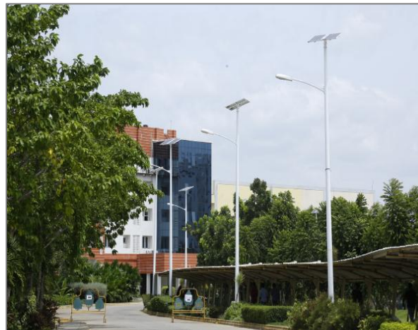
Solar panels powered exterior (pathway) lightings
