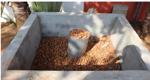
Rainwater Collection Pit
