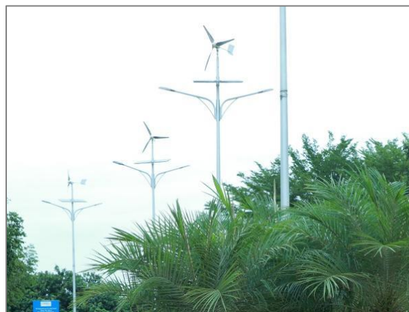
Wind-powered exterior (pathway) lightings
